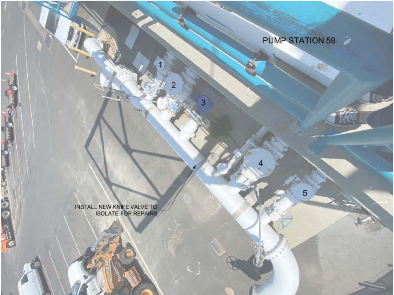
Image 2 – Pump Station 59 Outflows/Sewer Manifold
