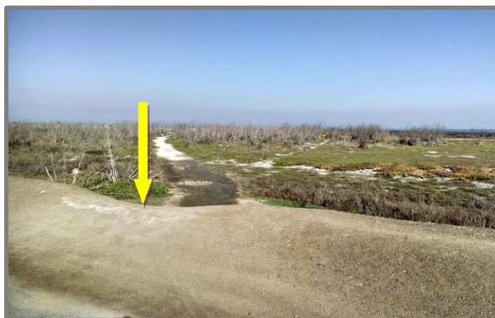
Figure 6-3. Foster City Levee Section with Levee Crest Compromised (yellow)
